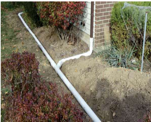
Down spout storm drains
