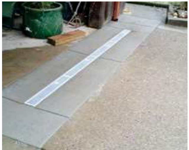
Surface trench drain
